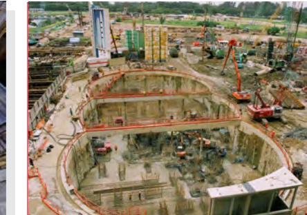
The Sail, Marina Bay Singapore Diaphragm Wall of 220m and thickness of 0.8m & 1.0m
